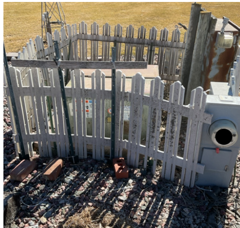
Customer added too much dirt which buried underground equipment, and there is not enough clearance from the fencing to the equipment.
