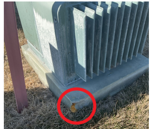
Mower hit and broke the fiberglass pad the transformer sits on. This allows rodents to enter and potentially cause damage.
