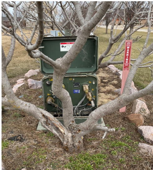
Shrub planted directly in front of the transformer. Minimum of 10' of clearance is required.
