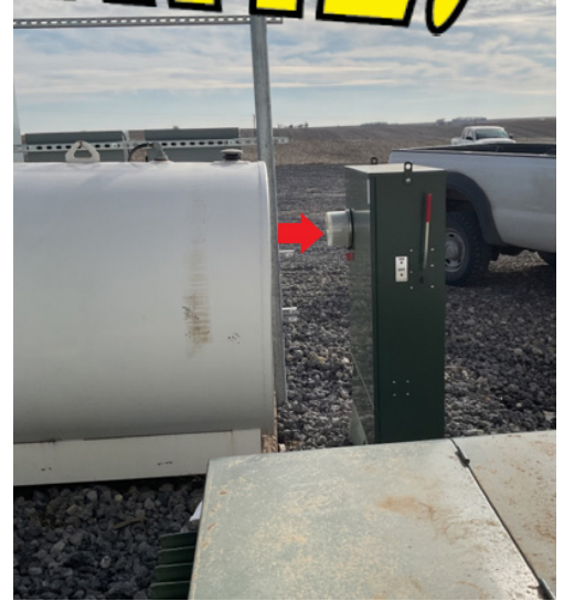
Fuel tank is too close to meter pedestal.
